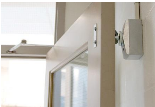
Figure 6.9: Electronic operated door hold-open device (floor or wall mounted)
